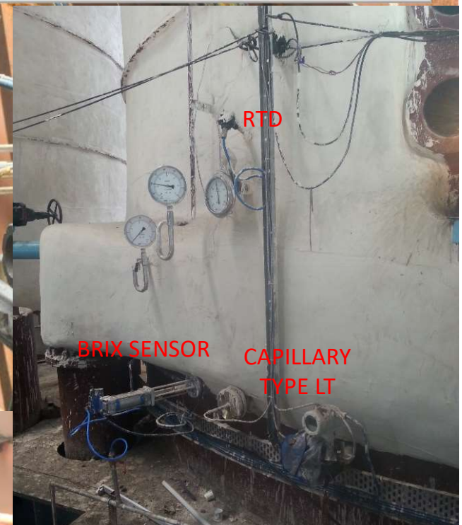
Brix, Capillary DPT Level, and RTD Temperature Sensor installed on Batch Type Vacuum Pan
