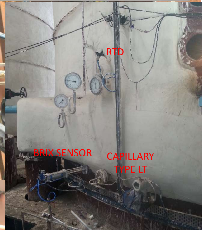
Brix, Capillary DPT Level, and RTD Temperature Sensor installed on Batch Type Vacuum Pan
